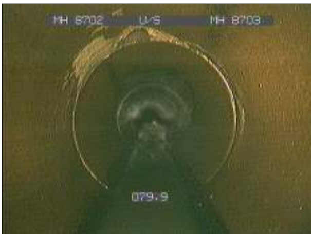
Photo: 283_25a, 00:06:54 79.9m, Hole in sewer at 12 o'clock, Remark: AT JOINT
