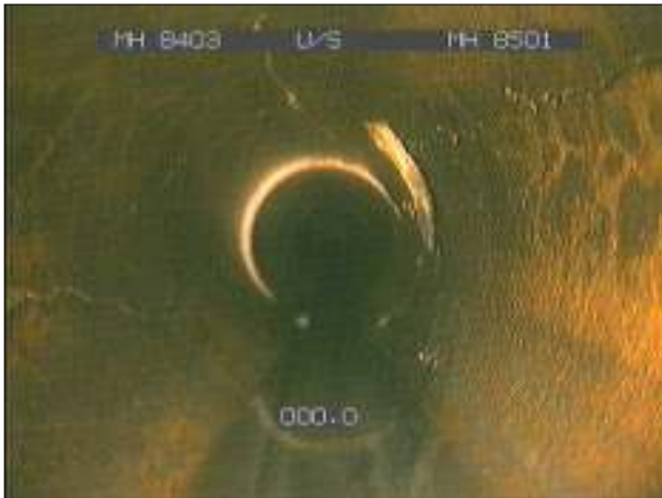
Photo: 151_4a, 00:00:00 0m, Longitudinal Fracture at 09 o'clock
