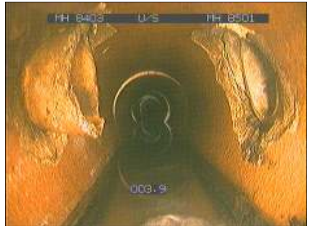
Photo: 159_12a, 00:01:21 3.9m, Connection, at 09 o'clock, dia 100 mm, intrusion 40 mm
