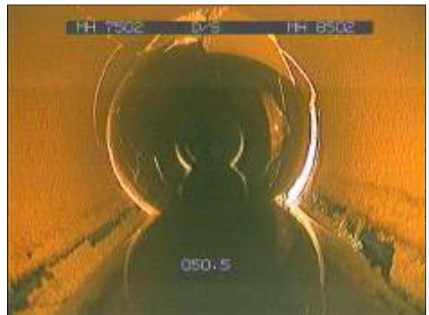
Photo: 4_35a, 00:06:35 50.5m, Sewer Broken, at 12 o'clock
