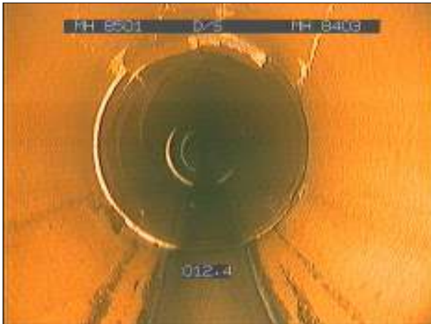
Photo: 5_18a, 00:02:49 12.4m, Hole in sewer at 12 o'clock
