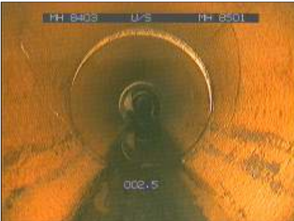
Photo: 158_11a, 00:00:56 2.5m, Circumferential Fracture, from 01 to 10 o'clock
