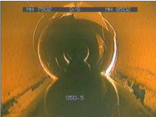
Photo: 4_36a, 00:06:40 50.5m, Circumferential Fracture, from 09 to 11 o'clock
