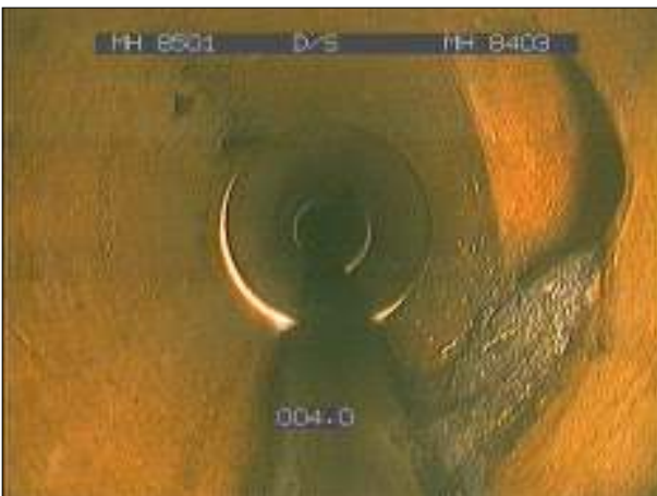
Photo: 5_10a, 00:01:04 4m, Encrustation light, from 03 to 05 o'clock, Remark: FROM JN
