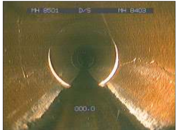
Photo: 114_6a, 00:00:30 0m, Longitudinal Fracture at 03 o'clock
