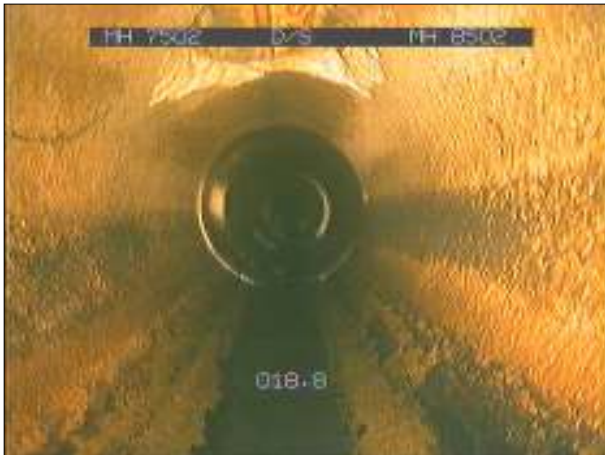
Photo: 4_12a, 00:02:11 18.8m, Hole in sewer at 12 o'clock
