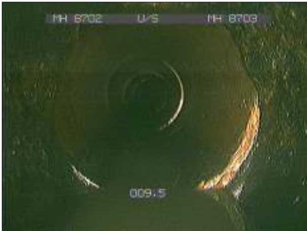
Photo: 267_9a, 00:01:34 9.5m, Joint displaced. Medium
