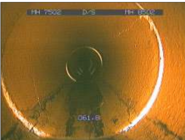
Photo: 4_45a, 00:08:39 61.8m, Longitudinal Fracture at joint at 07 o'clock
