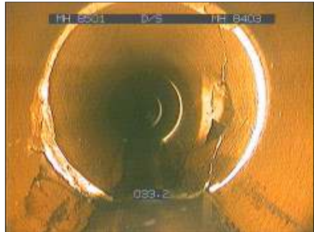
Photo: 139_30a, 00:05:47 33.2m, Circumferential Fracture at joint, from 01 to 05 o'clock
