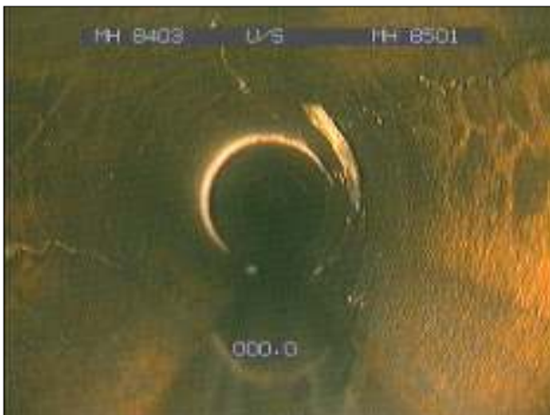
Photo: 153_6a, 00:00:00 0m, Longitudinal Fracture at 02 o'clock
