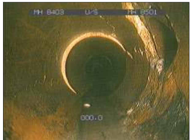
Photo: 154_7a, 00:00:19 0m, Circumferential Fracture at joint, from 03 to 05 o'clock
