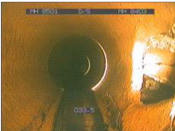
Photo: 140_31a, 00:06:03 33.5m, Connection defective, at 03 o'clock, dia 100 mm, Remark: INVERT MISSING IN CN
