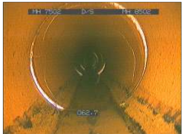
Photo: 4_47a, 00:08:54 62.7m, Circumferential Crack at joint, from 12 to 12 o'clock
