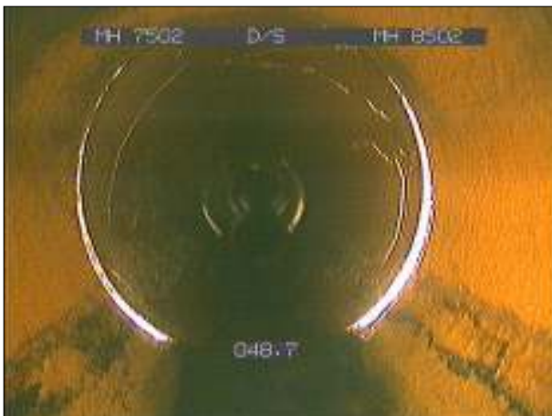
Photo: 4_30a, 00:06:09 48.7m, Multiple Fractures from 12 to 12 o'clock
