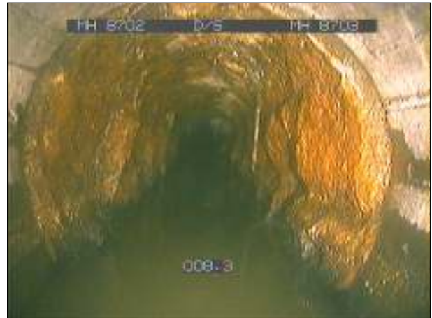
Photo: 248_6a, 00:00:53 8.2m, Encrustation heavy, from 07 to 05 o'clock, 25% cross-sectional area loss
