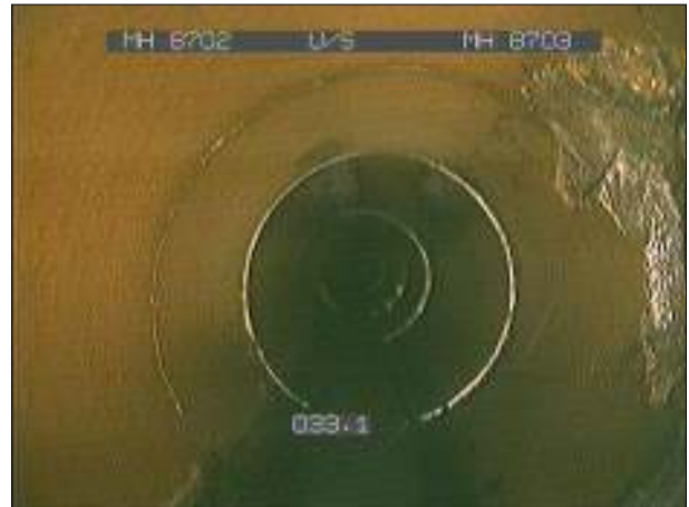
Photo: 274_16a, 00:03:28 33.1m, Circumferential Fracture, from 07 to 01 o'clock
