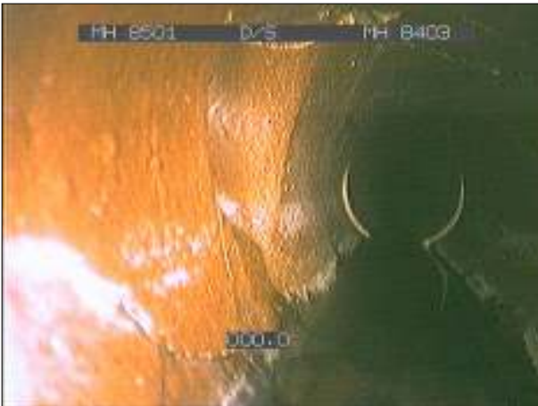
Photo: 112_4a, 00:00:17 0m, Circumferential Fracture, from 07 to 02 o'clock
