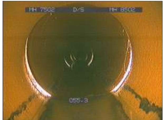
Photo: 4_41a, 00:07:26 55.3m, Circumferential Fracture at joint, from 03 to 05 o'clock
