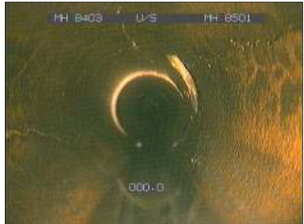
Photo: 152_5a, 00:00:00 0m, Longitudinal Fracture at 12 o'clock
