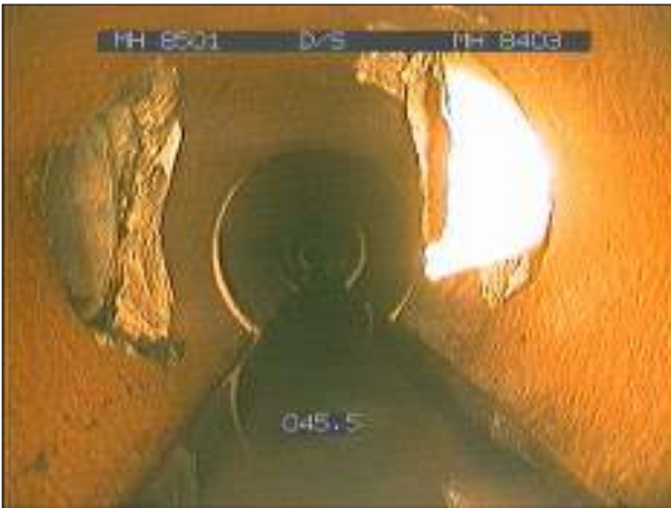
Photo: 145_36a, 00:07:32 45.3m, Connection, at 03 o'clock, dia 100 mm, intrusion 40 mm
