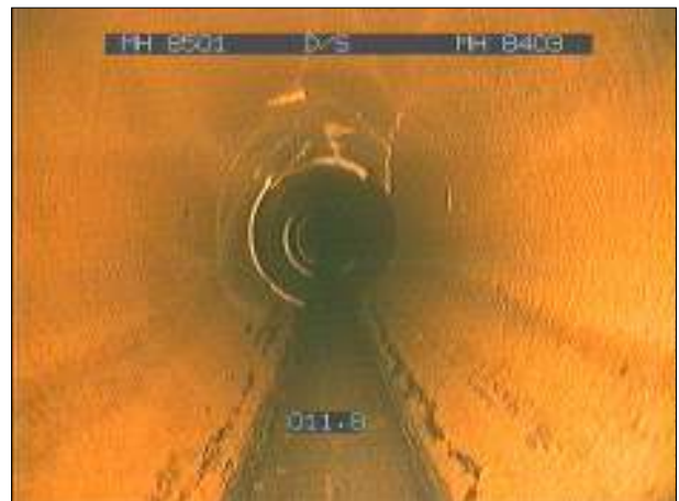
Photo: 5_17a, 00:02:15 11.8m, Multiple Cracks, from 08 to 04 o'clock
