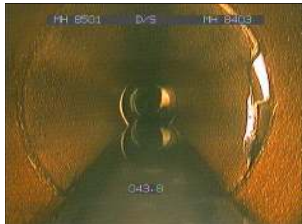
Photo: 144_35a, 00:07:19 43.8m, Hole in sewer at 03 o'clock
